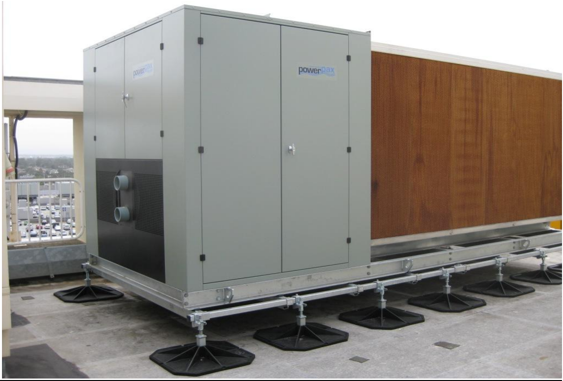
Images of Chiller in situ
